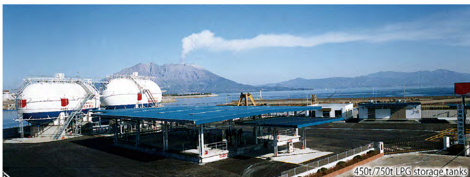
450t/750t LPG storage tanks
