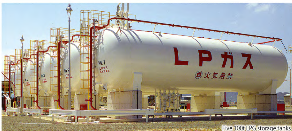
Five 100t LPG storage tanks
