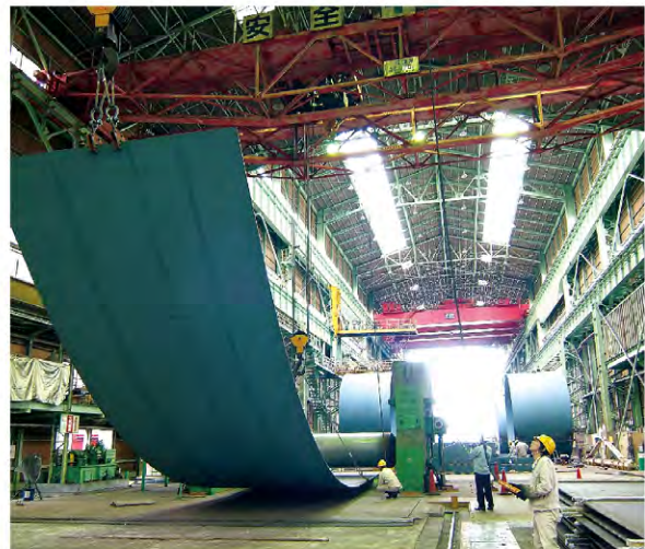
Shikoku Electric Power Co., Inc. Doigawa steel penstock stress contour display for FEM analysis
